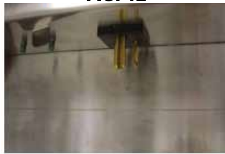
Fixed three prong connection
